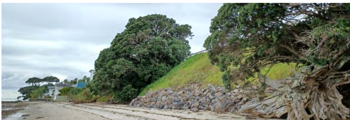
Figure 5-21: Cliffed section of road reserve showing a rock revetment installed in response to a coastal landslide
