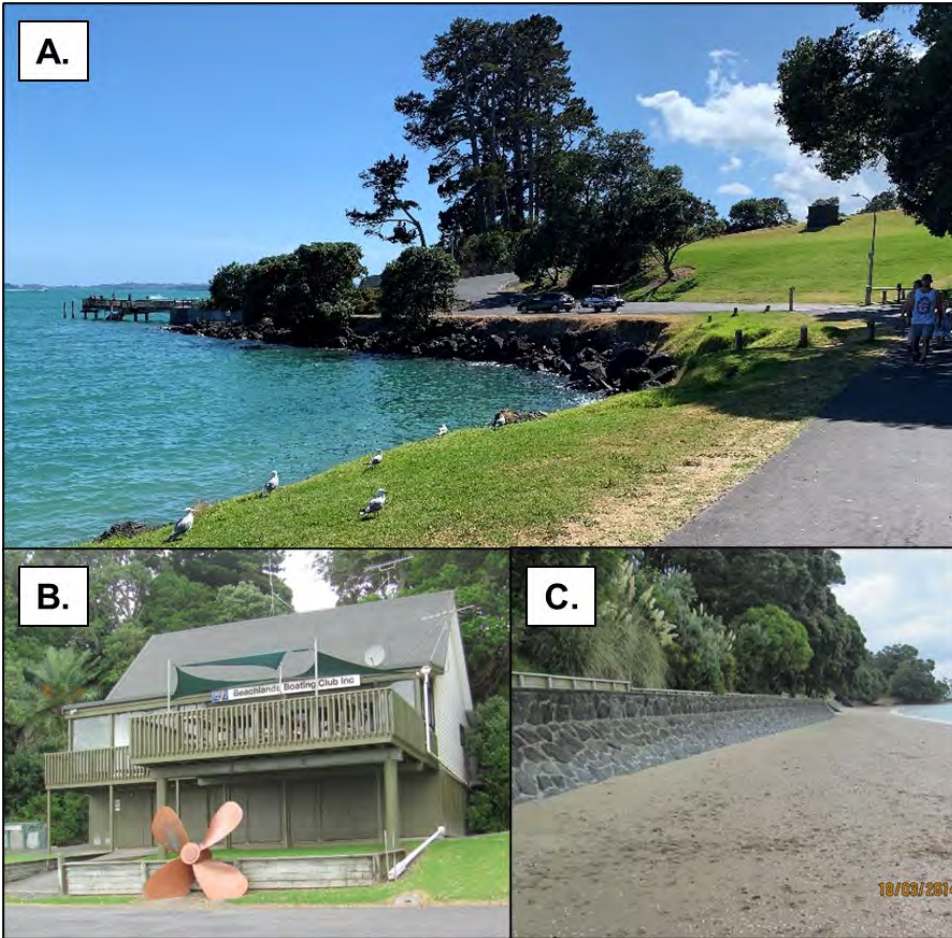
Figure 16: Photos of Sunkist Bay at high tide with top of revetment visible (A), the Beachlands Boating Club located along the foreshore (B), and the western seawall (C)
